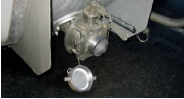
Bride borgne non installée
